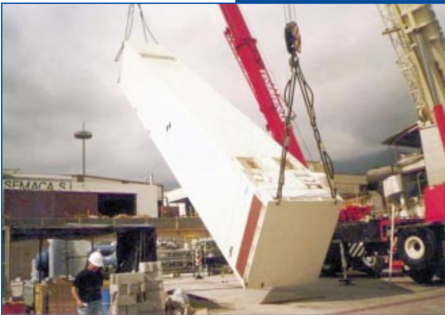
New ASPEN 1000 cold box being installed. The cold box houses the equipment that liquefies and distills the process air into liquid nitrogen, liquid oxygen and, optionally, crude argon. It also contains the main heat exchanger and distillation columns.
