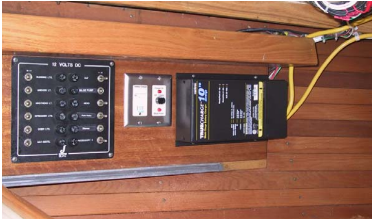
Rhapsody Electrical Control Area
