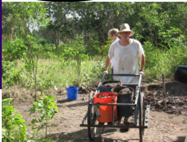
We recently were able to help Dulla mud wall his house. Jeremy is carrying mud from the pit (in background) over to the house.
